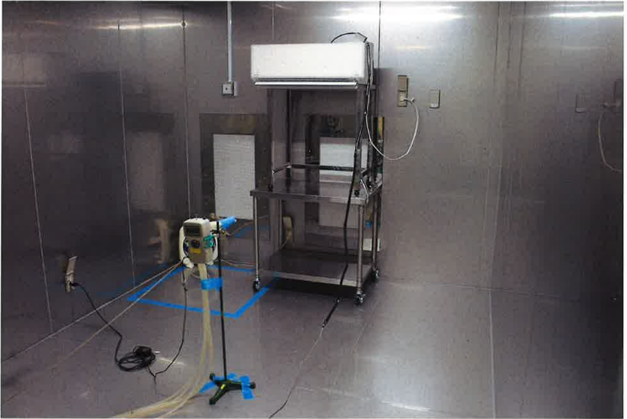
Photo 3. 25 m 3 Test chamber (Room air conditioner A)
